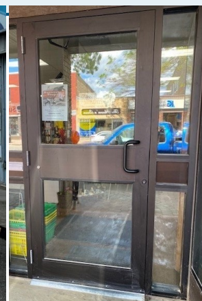
We contributed to the Almost New Store, who desperately needed to replace their front door.
